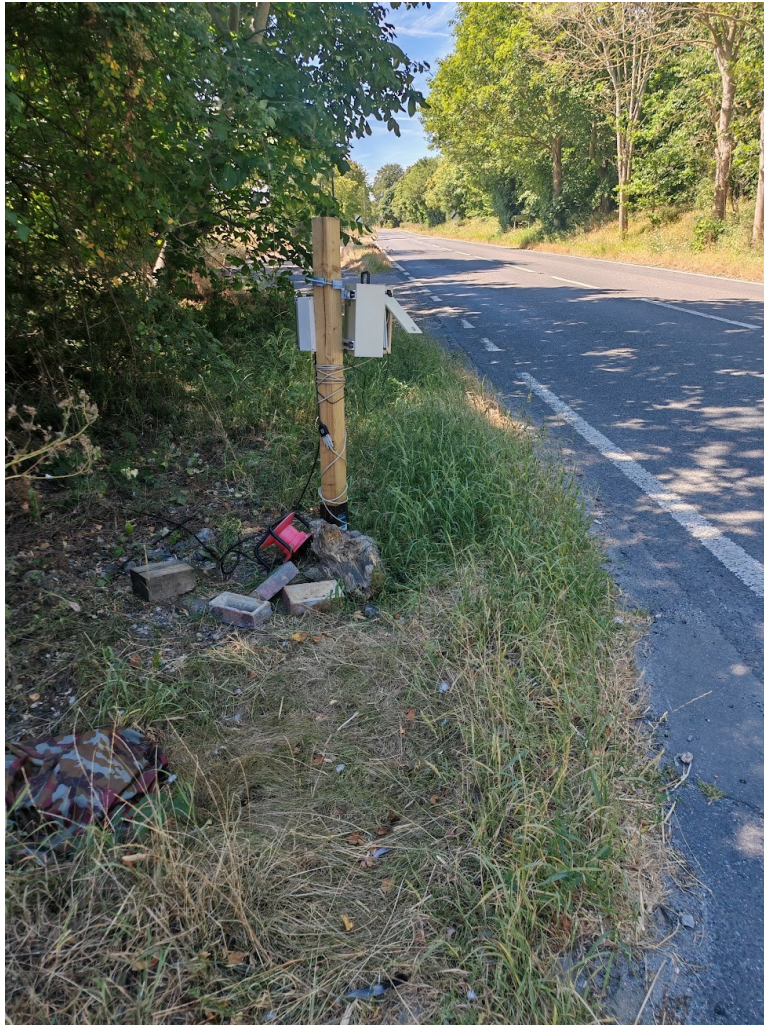
Figure 2: The ViaCount II installation at Fort George, Wickham Street. The radar sensor and data logger are mounted in the weatherproof enclosure on the timber post. The red unit at the base is the battery charger.
